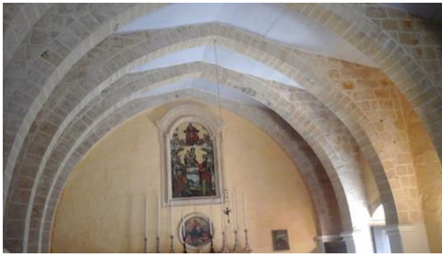
Figure 1: Early 15 th century Bir Miftuh Chapel Malta – 6.7m span X 14.5m depth X 6.7m height.
