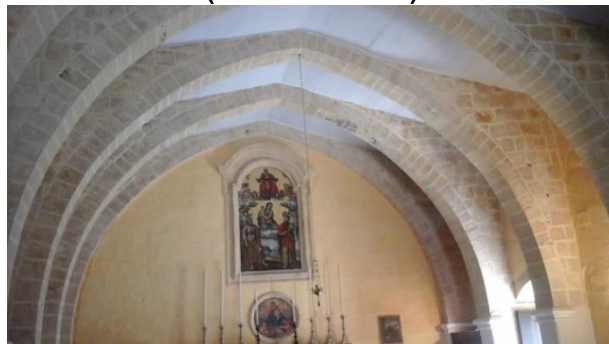
Figure 7: Chapel of Bir Miftuh in masonry construction in Gudja, built circa 1430: 6.7m width, depth 14.5m on a 6.7m height – stone slabs spanning 2.15m onto masonry pointed arches (SOURCE: Author).
