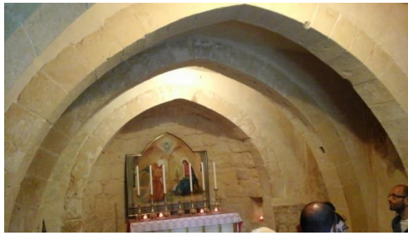
Figure 6: Chapel of Hal-Millieri in masonry construction Mqabba, consecrated 1480: 4.5m width, depth 7.5m on a 3.6m height – stone slabs spanning 1.525m onto masonry ashlar pointed arches, note rubble infill walling panels (SOURCE: Author).
