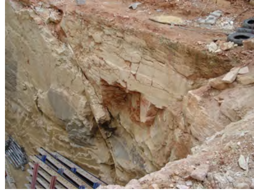
Figure 12.4: Badly fractured rock
