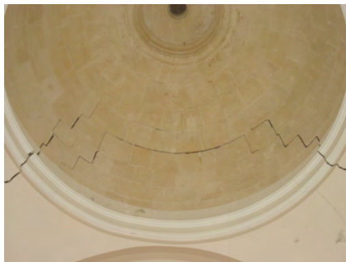
Figure 1.2: Cracks in the dome of Sliema Chapel
