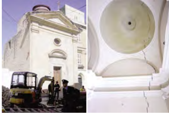
Figure 1.1: Picture of Sliema church and picture of cracks in dome.
