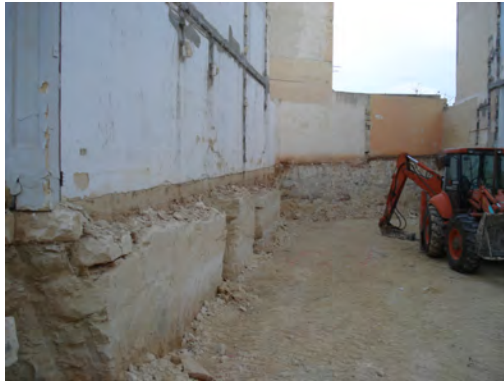
Figure 12.1: 0.75m away from party wall.
