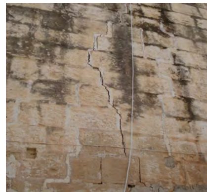
Figure 1.3: Cracks on façade of neighboring property.
